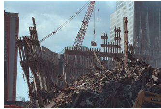
P8049-02 [Hi_j0050_2.JPG] 10/3/2001 VIEWS OF GROUND ZERO
