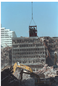
P8049-12 [Hi_j0040_1.JPG] 10/3/2001 VIEWS OF GROUND ZERO
