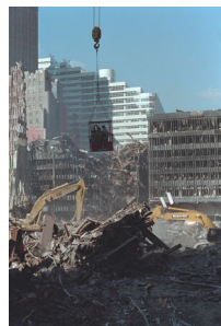
P8049-13 [Hi_j0039_1.JPG] 10/3/2001 VIEWS OF GROUND ZERO
