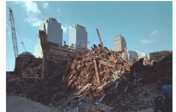
P8045-18 [Hi_j0052_1.JPG] 10/3/2001 VIEWS OF GROUND ZERO
